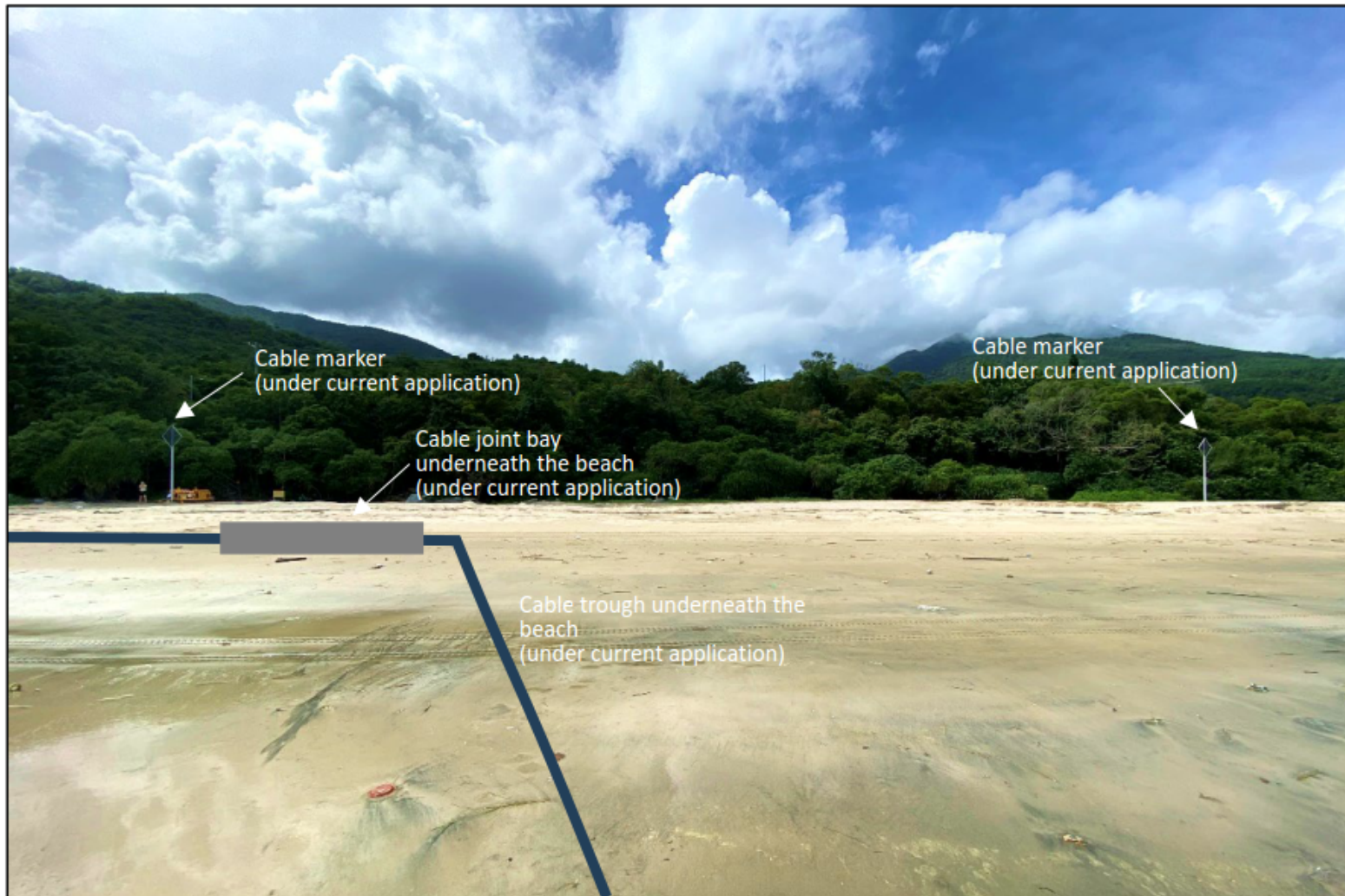
Plate 1: Site Photo of Cable Joint Bay, Cable Duct, Cable Trough and Cable Marker
